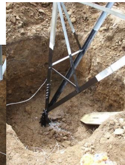
Pylons of ICE (Costa Rica)
