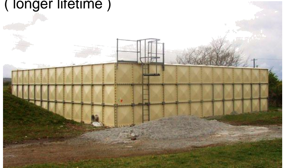
UK, Braithwaite tanks for potable water
